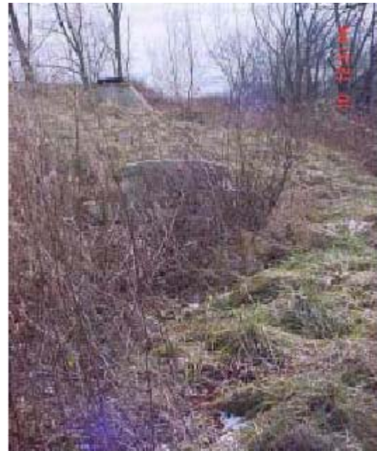
This trench has a subsurface energy dissipator to reduce the velocity of entering stormwater.
